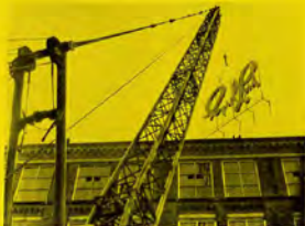
Raising a 20 foot sign 100 feet high, on the Cyril Lord Textile Factory near Oldham presented some interesting problems to Astley installation engineers. Our front page shows this sign in action at night.
